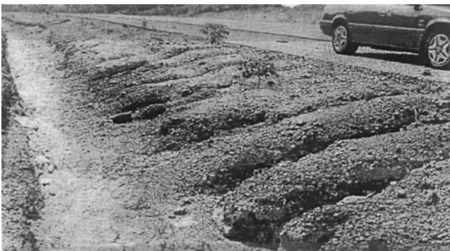
Fig. 2 Erosional rills created in the poorly compacted verge area along the highway
