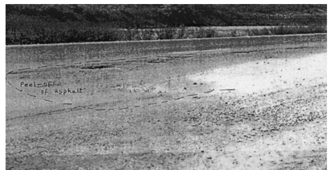
Fig. 4 Typical separation/peel-off of asphalt finish
