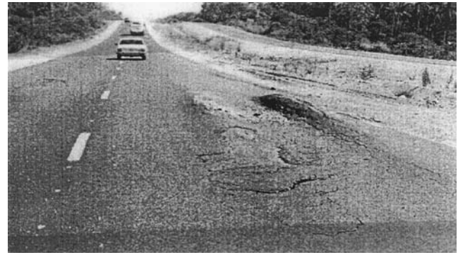
Fig. 3 Typical failure of asphalt finish by localized subsidence and distortion
