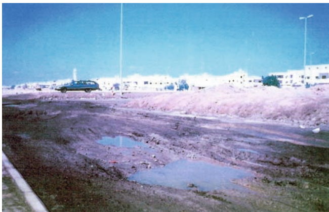
Fig. 3 Photograph showing subsidence pits in the pavement due to subsoil wetting in north Jeddah city
