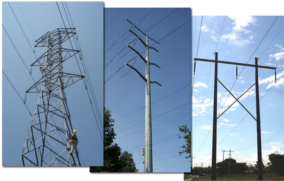
Fig. 1 Structures for high-voltage electricity distribution: steel tower, tapered steel pole, H-type structure
