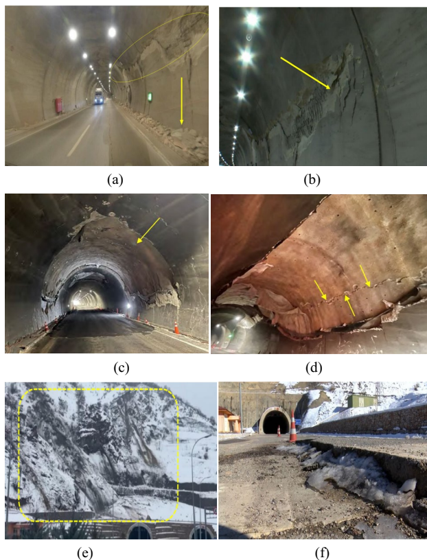
Fig. 9 a, b Spalling of concrete linings, c a portion of the roof and sidewall damage, d longitudinal cracking, e traces of rockfall above the portals, f pavement dislocation at the entrance of the portal (Source: GEER and EERI Report 2023; Aydan and Ulusay 2023)
