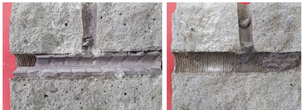
Fig. 12 High-quality encapsulation (left) around fibre glass bolt (right) around the concrete medium
