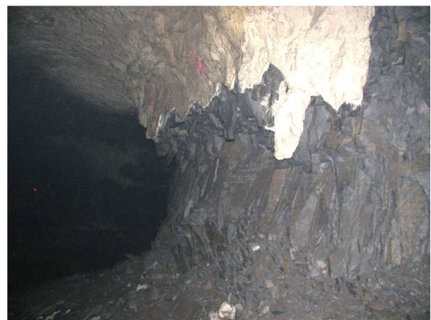
Fig. 1 Time-dependent scaling of a manganese pillar in a hard rock bord and pillar mine in South Africa. The pillar was covered with thin spray-on liner to prevent the scaling, but the ongoing failure destroyed the liner and the scaling continued
