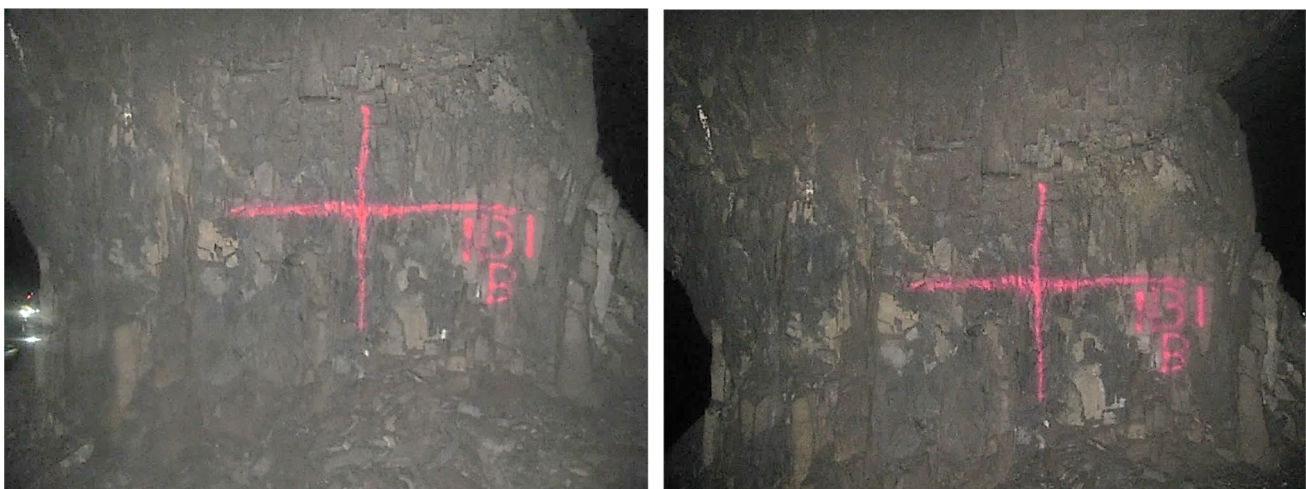
Fig. 4 A measurement cross painted on a manganese pillar. The photograph on the left was taken on 6 May 2021 and the photograph on the right on 18 August 2021. The lines were still pristine on the second date and no scaling occurred during this 3-month period
