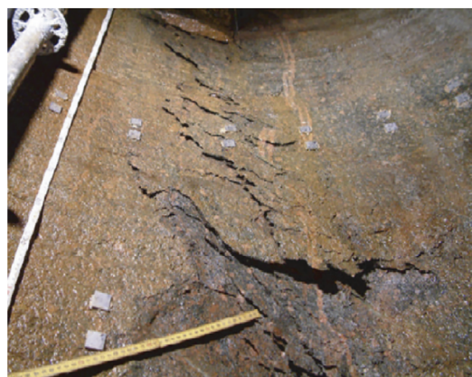
(b) Spalling failure (Martin and Christiansson, 2009)
