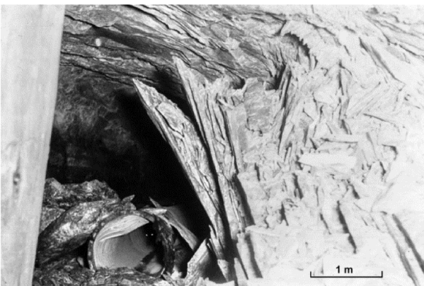
(b) severe rock failure in an access tunnel (Hoke 2014)
