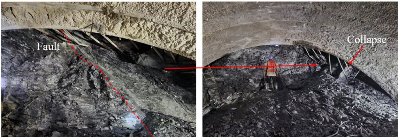
Fig. 3 Surrounding rock collapse at fault
