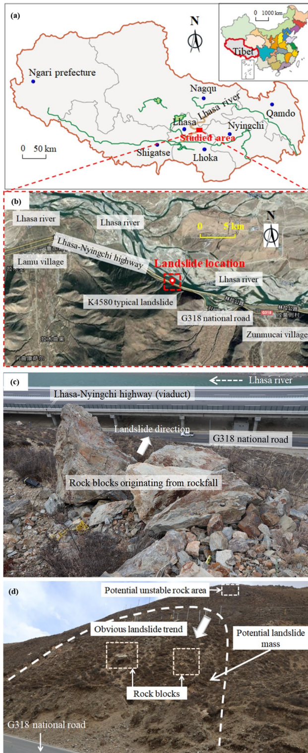
Fig. 1 K4580 typical slope along the G318 national road in Tibetan Plateau. a Studied area, b landslide location, c photo of the scene, and d photo of the slope
