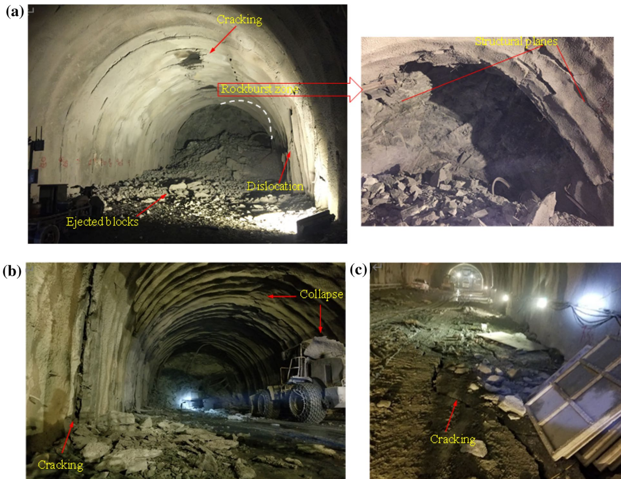
Fig. 8 Rockburst and damage characteristics of the Micangshan tunnel
