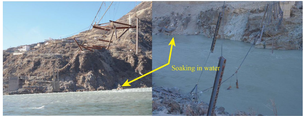
Fig. 1 Rock mass soaking in water, examples of bridge along the Jinsha River in Yunnan, China
