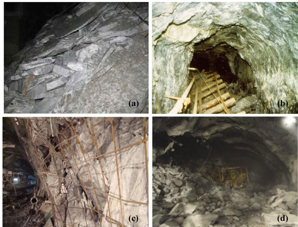
Fig. 1 Typical failure modes of hard rock near deep excavation: a spalling/slabbing (Gong et al. 2012), b floor heave (Cai and Kaiser 2018), c buckling, and d rockburst (Zhang et al. 2012)
