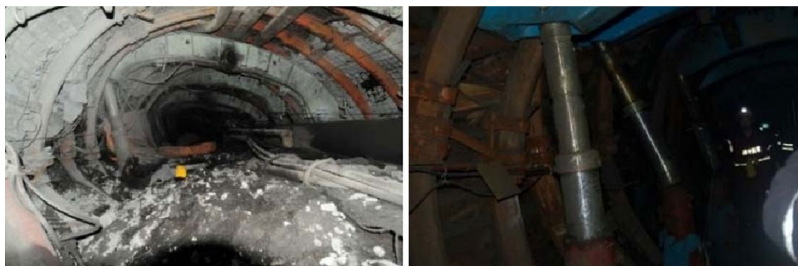
Fig. 1 Damage of the roadway caused by a rock burst
