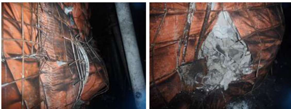
Fig. 2 "Bulging" deformation phenomenon occurs in the RBB
