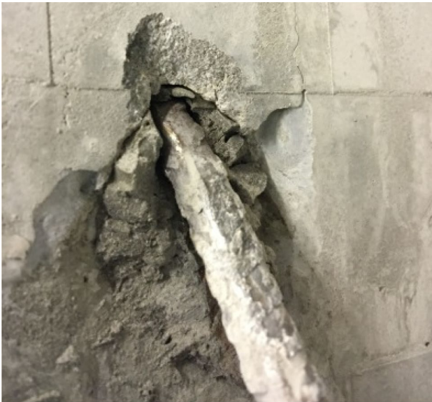
Fig. 16 Concrete was crushed around the joint intersection for inclined 8-mm rockbolt
