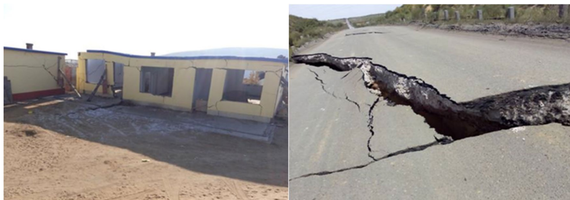
Fig. 2 Damage to buildings and roads in mining areas
