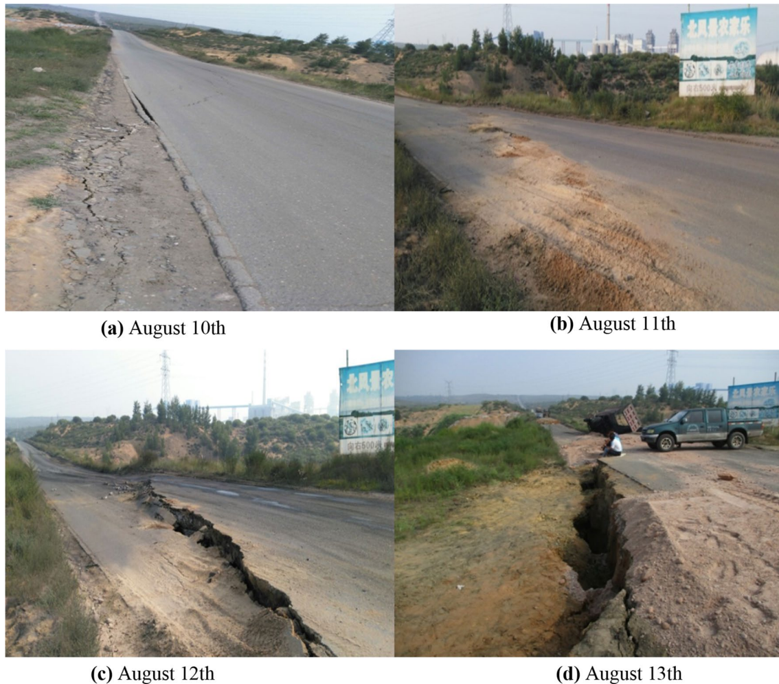
Fig. 17 Crack CLF1 variation process. a August 10th, b August 11th, c August 12th, d August 13th
