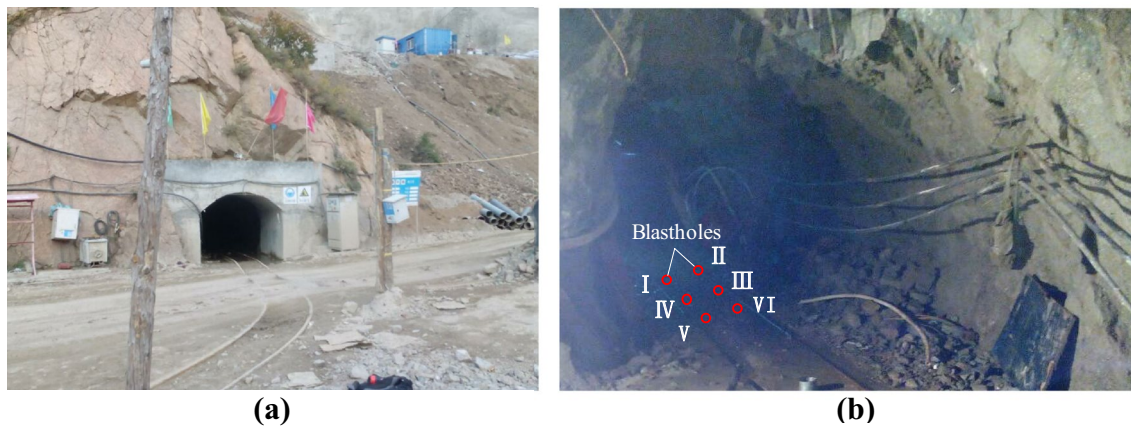
Fig. 13 Site description of the case study in Fengning pumped storage power station: a geology exploration tunnel; b test area and onsite layout of blastholes
