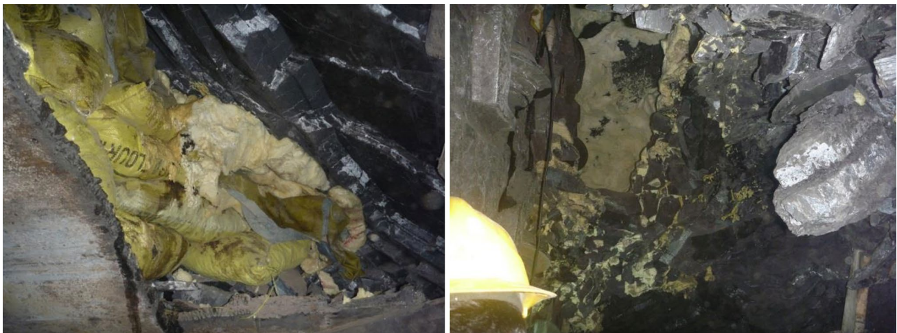
Fig. 25 Two-component foams injected through the collapsed blocks in front of the cutterhead
