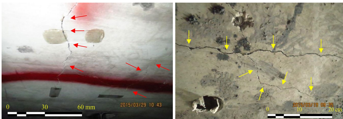
Fig. 15 Formation of longitudinal cracks in roof segments in the chainage 18+498 km to 18+546 km
