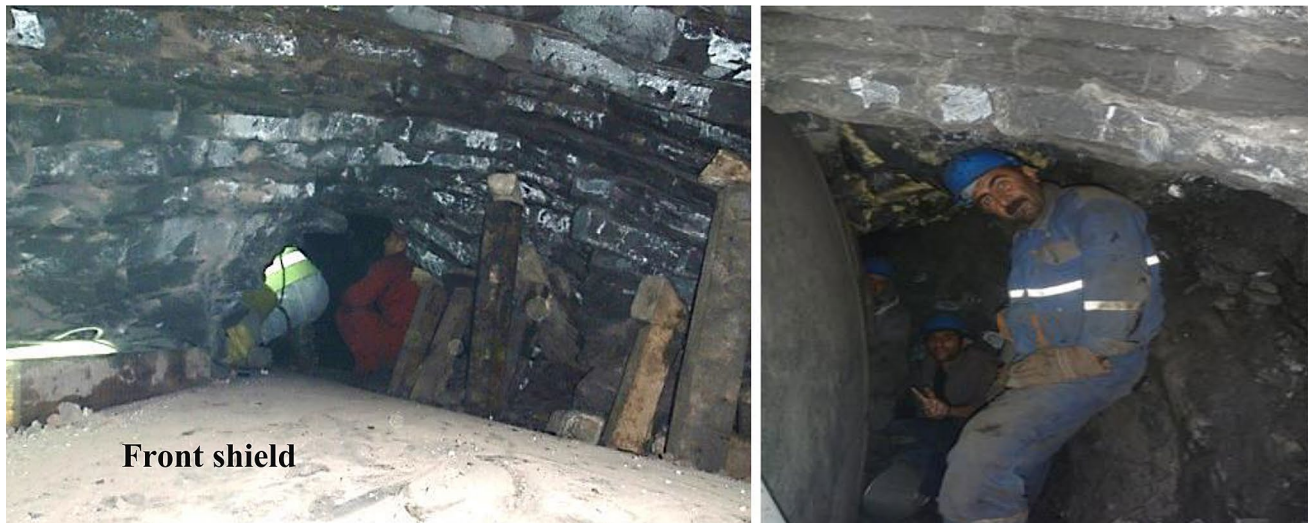
Fig. 23 Excavation operation and the gallery in right and upper side of the front shield
