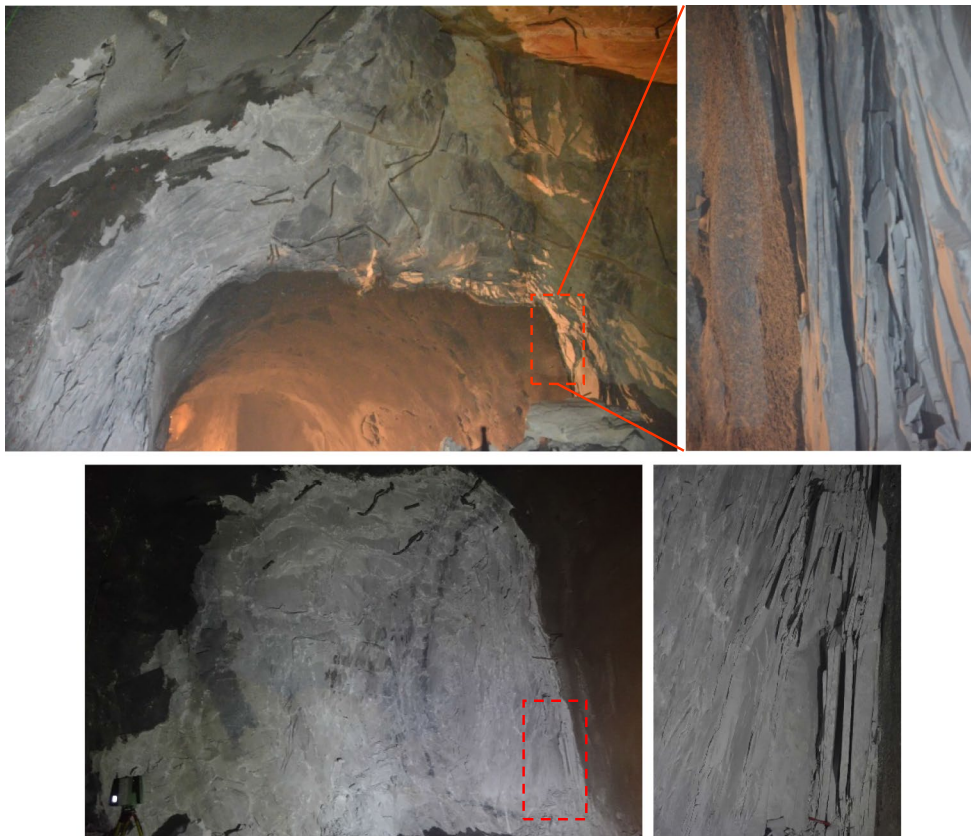
Fig. 5 Rock spalling occurred after slashing excavation of II b and II a at the 7# Lab
