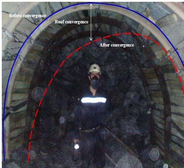
Fig. 7 Comparison of main gate roadway situation before and after convergence in Parvade-2 coal mine
