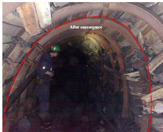
Fig. 6 Main gate roadway in Parvade-2 coal mine after convergence
