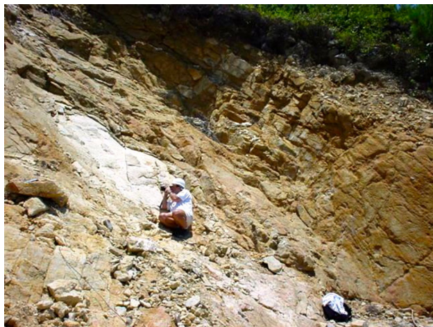
Fig. 27 Part of the failed area of the Leung King Estate landslide. The upper, darker rock mass is fractured and deteriorated; the light central area is the upper part of a sheet joint above which progressive movement had occurred over many years
