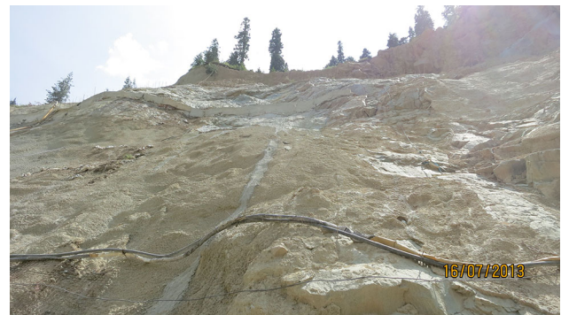
Fig. 36 Larger scale waviness (first order). The temporary fence (about 1.5 m in height) about half way up slope and the hose in the foreground follow the joint waviness undulations
