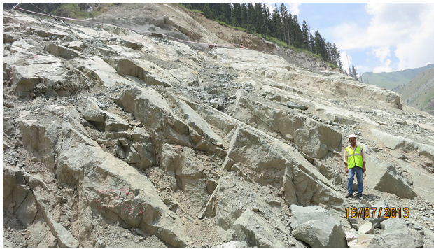
Fig. 32 View along strike of set of daylighting discontinuities
