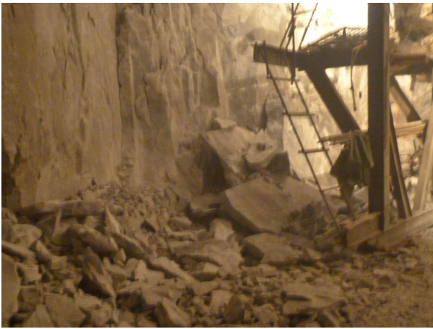
Fig. 9 A moderate rock burst occurred at Stake K5 + 623 – 628 in the drainage tunnel on June 20, 2011
