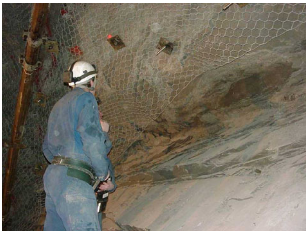
Fig. 2 View of a front with chevron fractures at the main level (from Geoter)
