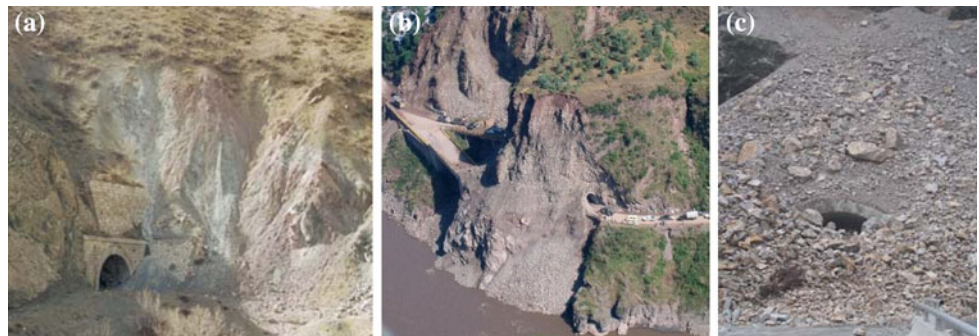
Fig. 21 Examples of damaged portals of tunnels. a 1992 Erzincan. b 2005 Kashmir. c 2008 Wenchuan
