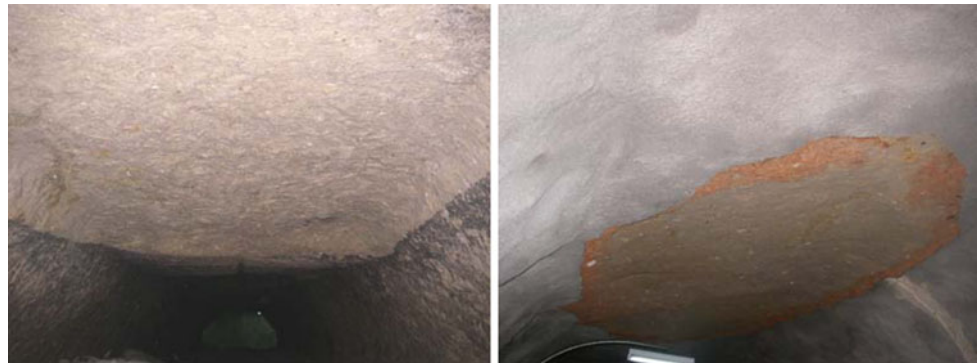
Fig. 20 Spalling from the roof in Bukittinggi underground shelter by the 2007 Singkarak earthquake
