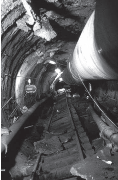
Fig. 6. Floor heave about 100 m behind the Intake drive TBM in 1979 at a depth of 400 to 425 m below surface
