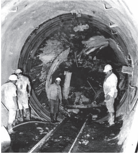
Fig. 7. Excavation of the remains of the TBM in 1987 during the fourth contract
