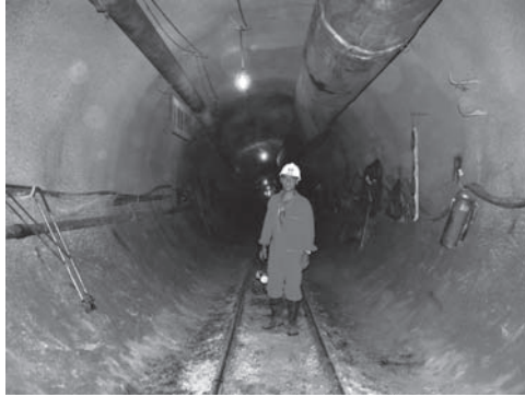
Fig. 25. Completed tunnel lining in one of the deepest sections between Chainages 10,000 and 12,000
