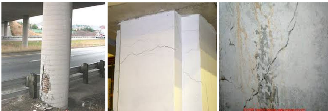
Fig. 1 Cracks in columns
