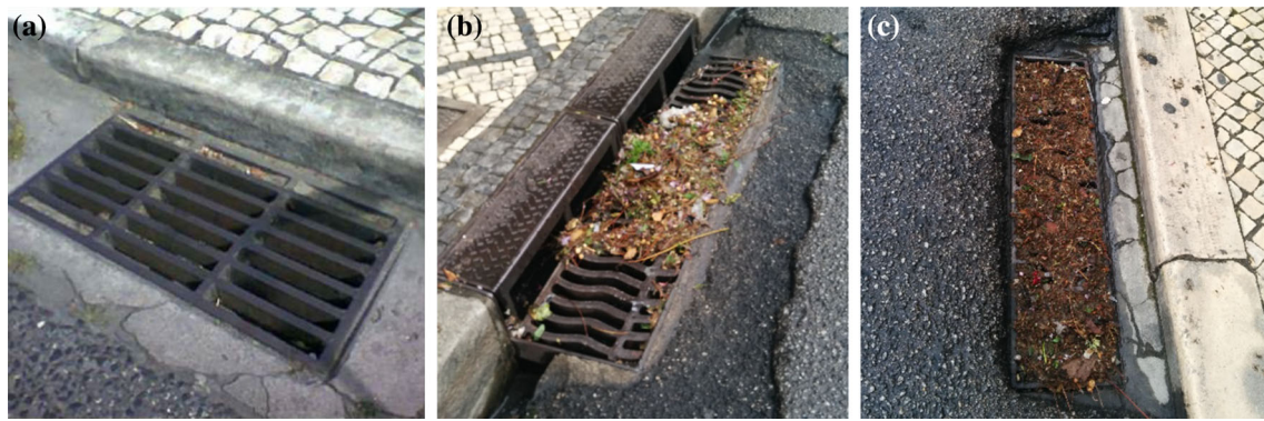
Fig. 1 Sewer inlet cleaning conditions. Images (b) and (c) were taken after a storm event on 15 April 2015 which caused flooding in the Praça 8 de Maio (Coimbra, Portugal). a Clean inlet grate, b partially
