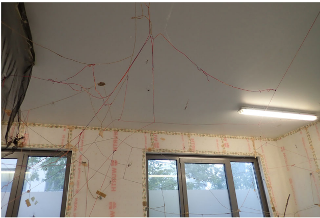
Fig. 12 Threads under the ceiling and damp-proof ceiling light
