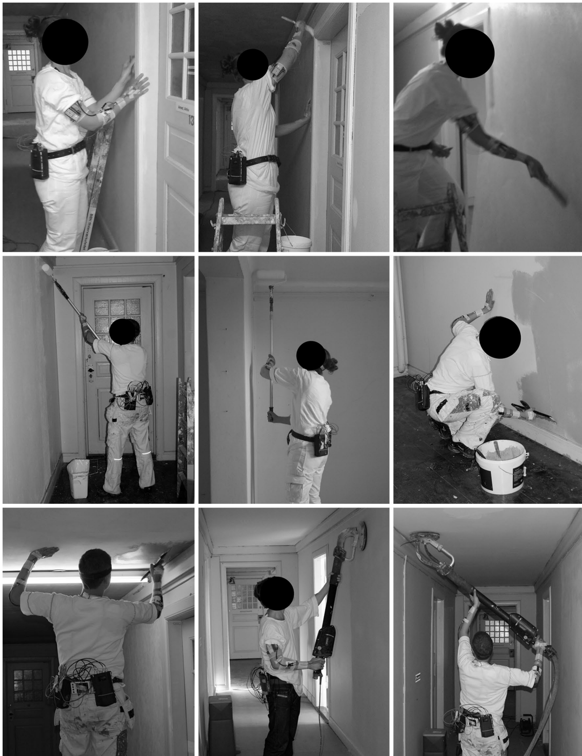
Fig. 2 The work tasks investigated, from the top left : Sanding (by hand); painting (brush); mounting glass felt; painting wall (roll); painting ceiling (roll); full levelling, wall; full levelling, ceiling; sand-
