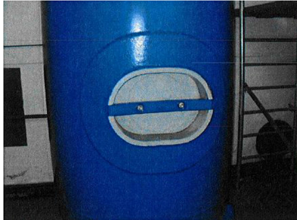
Fig. 3 The pressure vessel with the manhole cover
