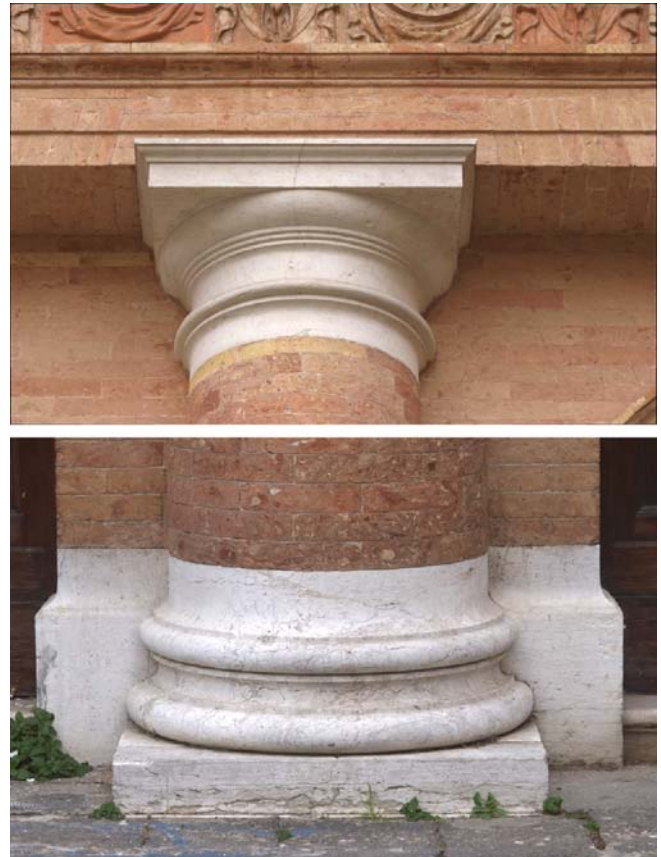
Fig. 24. Ambiguities between the vocabulary of the architect and physical divisions of the elements
