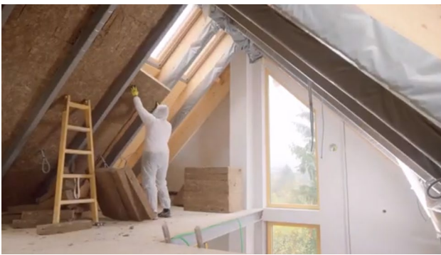
Fig. 3 Using cork palates in a building to reduce the energy losing and noise
