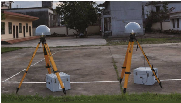
Fig.3 The continuously-operating GPS station
