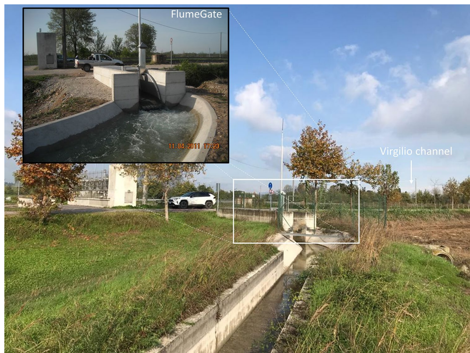
Fig. 2 The FlumeGate installed at Ponte Trento diversion point
