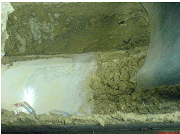
Fig. 6 Muddy material resulting from EPBM
