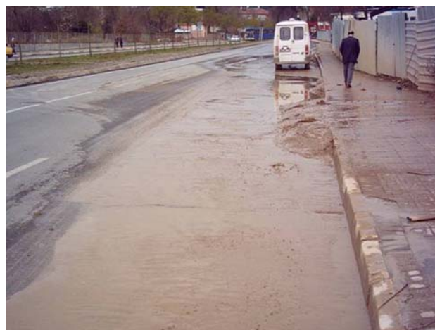
Fig. 11 Mud that has spread over Eyüp Aksoy Street during the Kadıköy–Kartal Metro excavation
