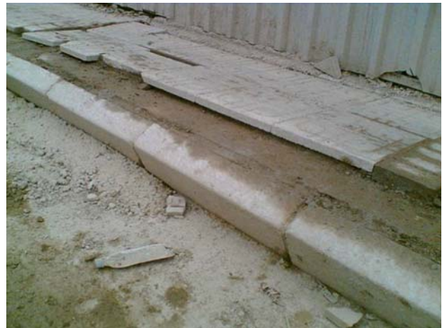
Fig. 13 Deformation that occurred in the pavement during the Kadıköy–Kartal Metro excavation
