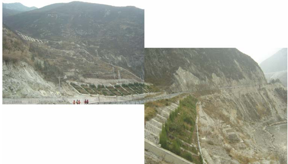
Fig. 3 Photograph of the Xiaozongqu landslide showing the geomorphology, the road, the landslide and the repaired slope
