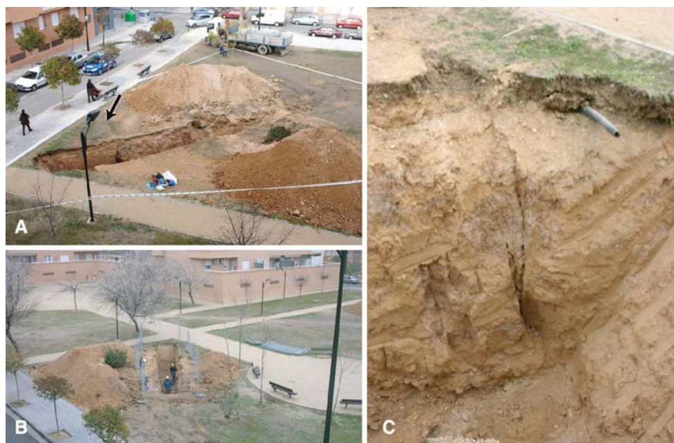
Fig. 8 a View of trench SW. Arrow points to the scarp affecting the recent artificial soil. b View of trench SE2. c Open cracks in the SE wall of Trench SW, next to its southwestern edge. Images taken on January 2008
