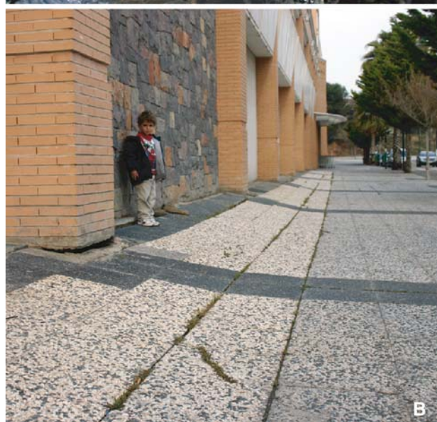
Fig. 4 a Opened joint in the upper part of the building showing a main longitudinal displacement and a secondary transverse displacement component (Photograph taken on March 7, 2008). b Tilting and cracking caused by subsidence next to the stable building A (Photograph taken on April 2007)
