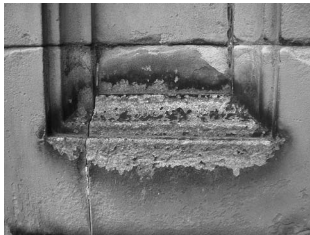
Fig. 2 Pitting of this sandstone is caused by subsurface growth of organisms. Decay is confined to the area which is most commonly wetted by rainwater
