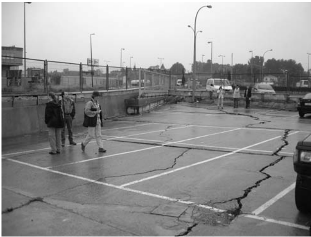
Fig. 3 Fractures developed in the parking lot of a factory in the northwest of Zaragoza
