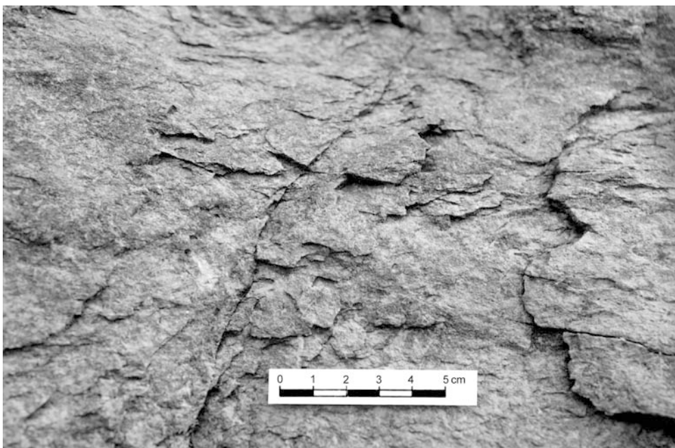
Fig. 11 Weathering form “multiple flakes to crumbling (mF-Pu)”
