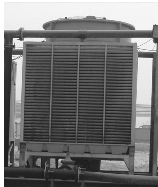
Fig. 6 A view of a cooling tower without sunshade
