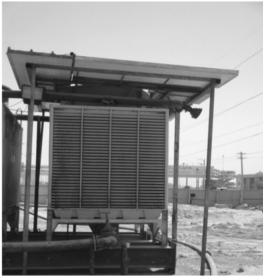
Fig. 7 A view of a cooling tower with sunshade
