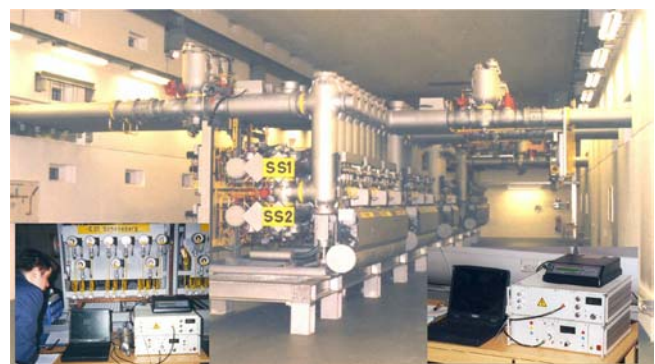
Fig. 3 Making ion mobility spectrometer measurements at a German gas insulated substation
