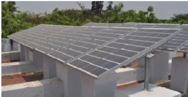
Fig. 16 Solar Plant of rating 1kWp
