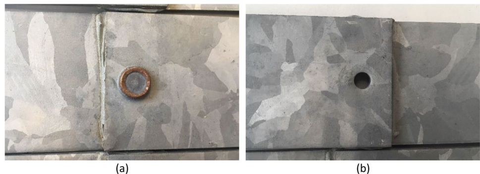
Fig. 11 Example of an HDG-Zn hybrid joint specimen after 2 years of outdoor exposure: a corrosion on the die side, and b unaffected punched side
