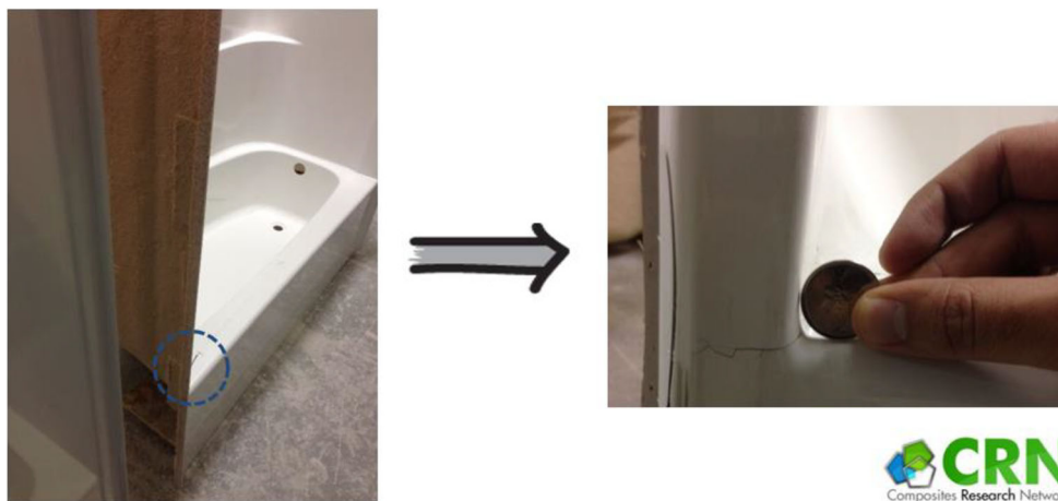
Fig. 3 Example of a corner crack defect, seen in tub showers after de-moulding
