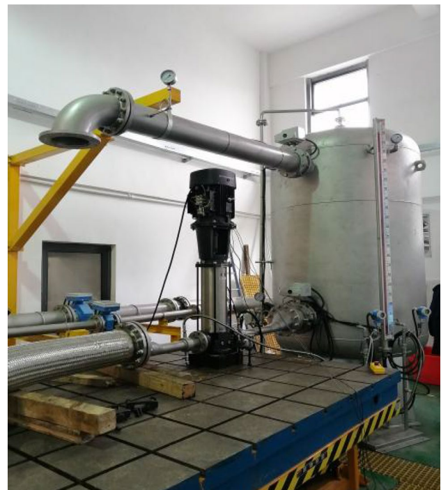
Fig. 3 Pump test facility
