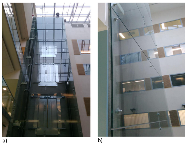
Fig. 1 Suspended glass panels utilized as external walls for a lift system in Tallinn University of Technology. a Global view. b View of one of the rectangular suspended panels of the façade
