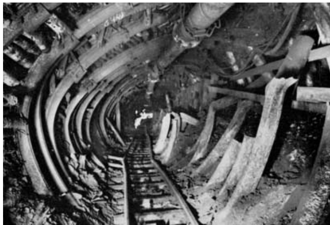
Fig. 7 View along strike of active thrusting exposed in a mine near Peissenberg in subalpine molasse, north of the Alps, triggered through mining at about 1,120 m below ground. Figure courtesy of Mrs H. Illies (Illies and Greiner 1976)
