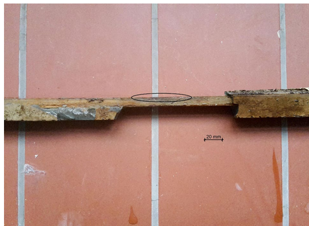
Fig. 13 Top view of the “12 months CEM” sample with initiating deterioration in regions with low cement covering (elliptical marker)
