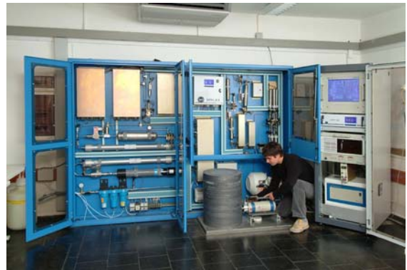
Figure 4 SPALAX noble gas system installed at the Radionuclide Station RN33 at Schauinsland, Germany
